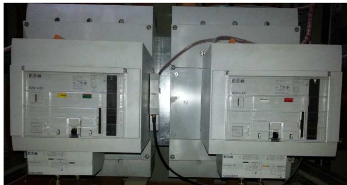
Figure(3.6): Indoor of ATS board in electrical distribution board
