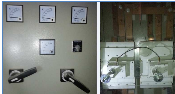
Figure(3.4): Indoor and Outdoor of MTS board in electrical distribution board
